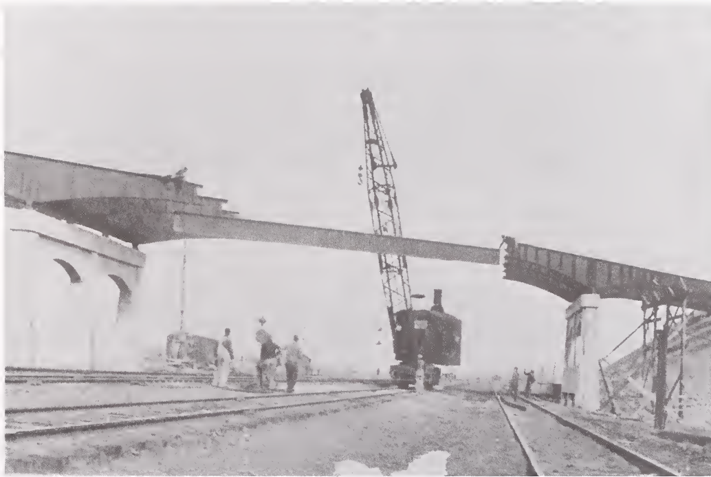
Setting the middle girders of the Mossmain overpass, 1936 (Photograph courtesy of Bob Robbins).
